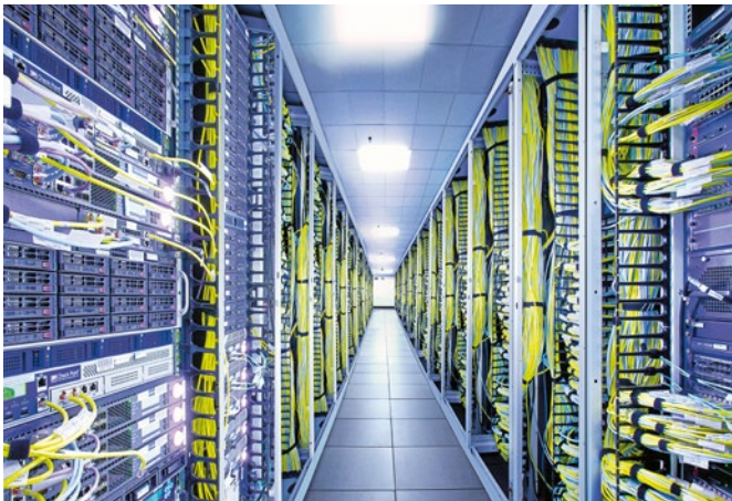
Demanding data center application
